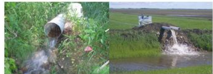
Free flowing tile outlet and a pumped outlet
