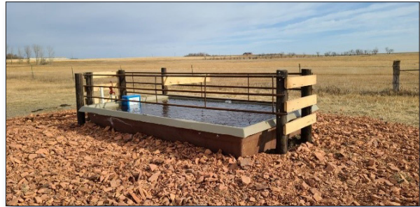
Figure 2. A producer installed this watering tank using CWA section 319 funds.
